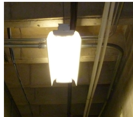
Interior light fixture in York County Courthouse to be replaced with grant funding from the Nebraska Energy Office.
