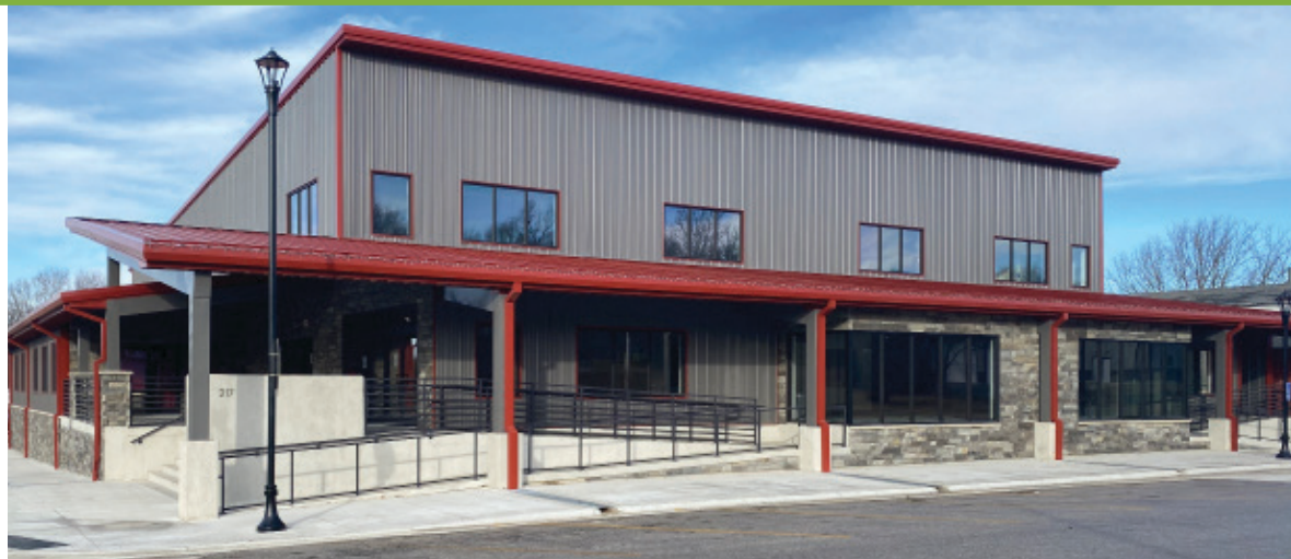
(Above) Reconstruction of the Nebraska Communities Playhouse, which helped remove architectural barriers and material that restricted the accessibility opportunities for persons with disabilities.
